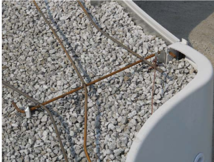
Photo B4 – A conductive mesh below the deck in solid contact with the pool
